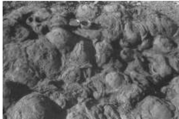
Fig.6.4 : Exfoliation (Flaking) and granular disintegration
